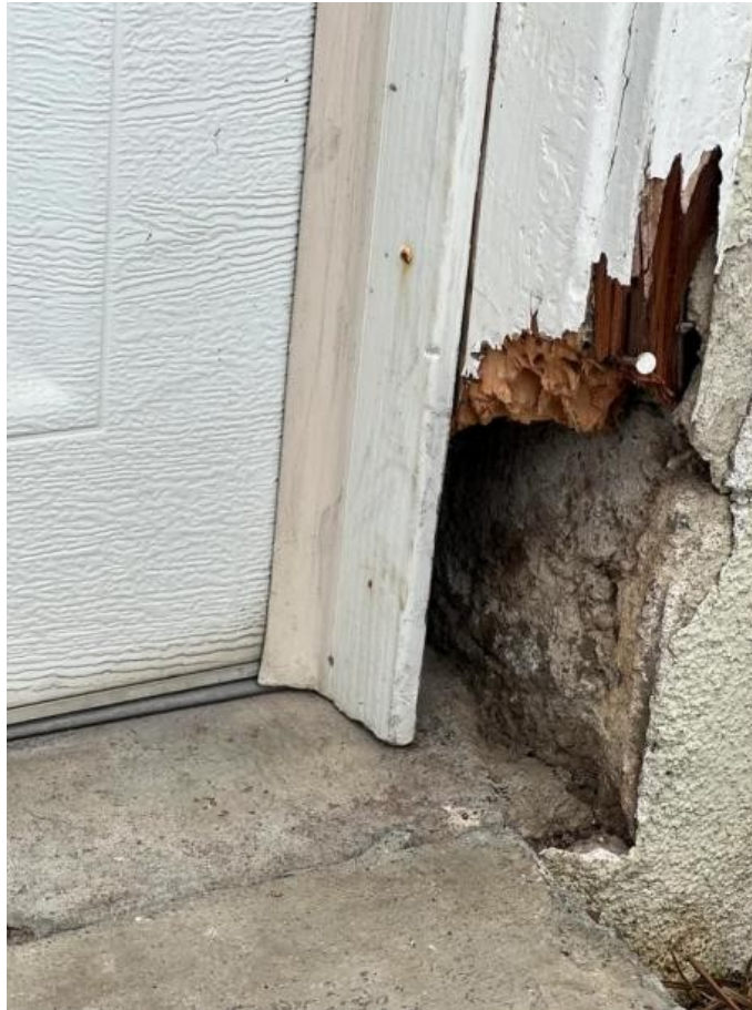
Rot often starts low on the casing where water can sit against wood and masonry.
